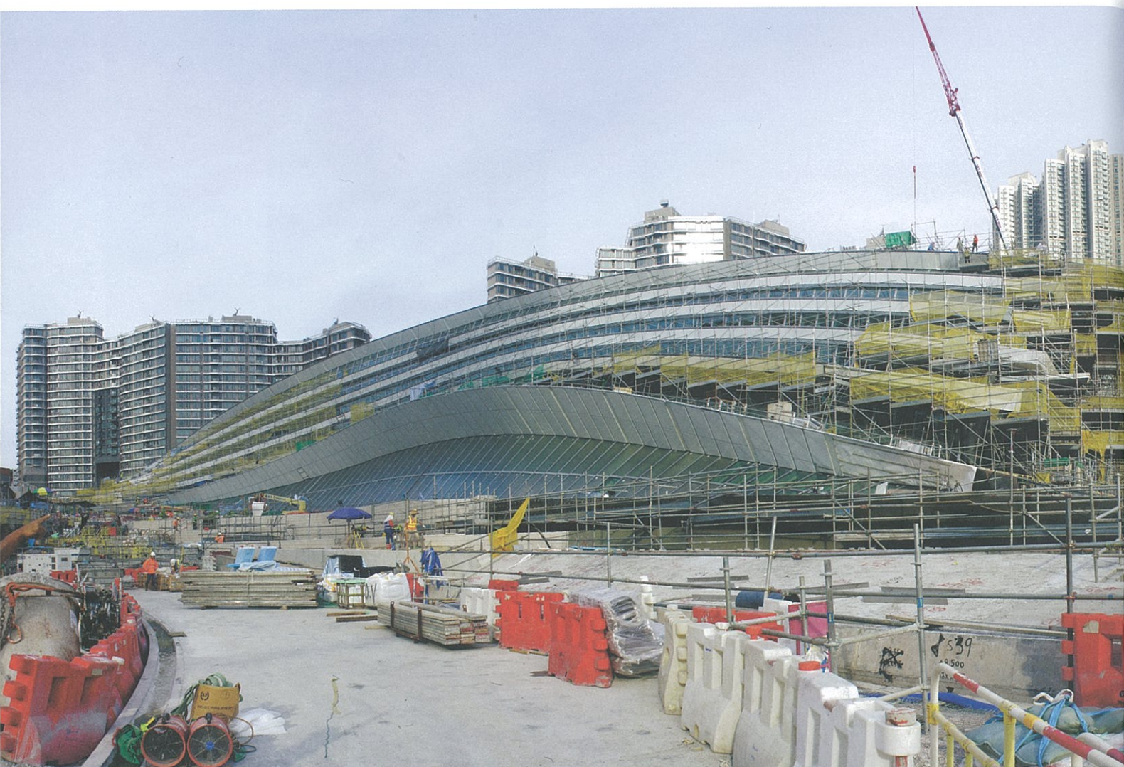
The construction scene of West Kowloon Station, photo taken on 6 October 2017. When it opens at the end of 2018, the station is expected to serve 109,000 passengers a day
